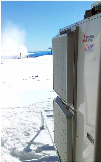
Ecodan Hot Water Heat Pump Zubadan Series installed at "The Lodge" – Ruapehu Ski Club.
